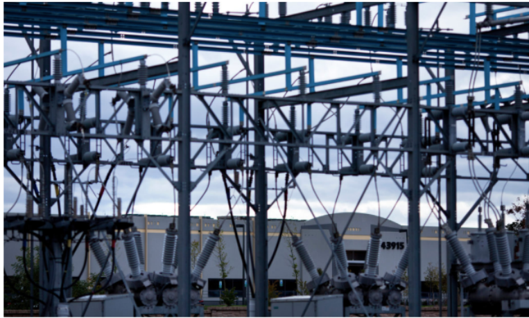
A NATURAL PAIRING A data center in Ashburn, Va., seen past a Dominion Virginia Power substation serving it. Worldwide, such centers use the rough equivalent of the output of 30 nuclear power plants. Brendan Smialowski for The New York Times
