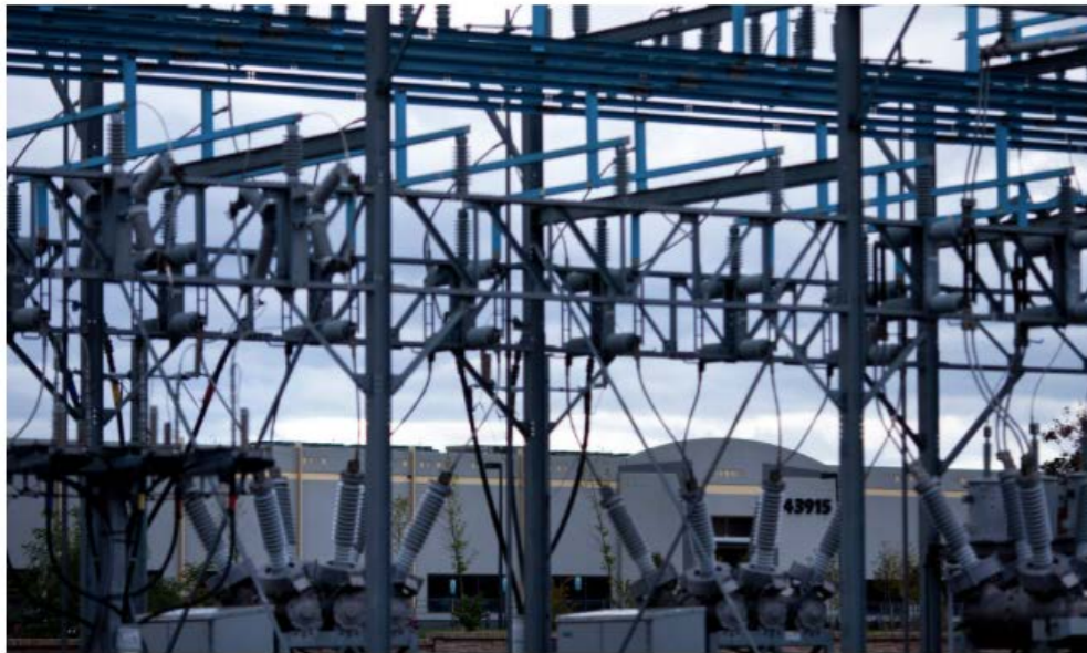
A NATURAL PAIRING A data center in Ashburn, Va., seen past a Dominion Virginia Power substation serving it. Worldwide, such centers use the rough equivalent of the output of 30 nuclear power plants. Brendan Smialowski for The New York Times
